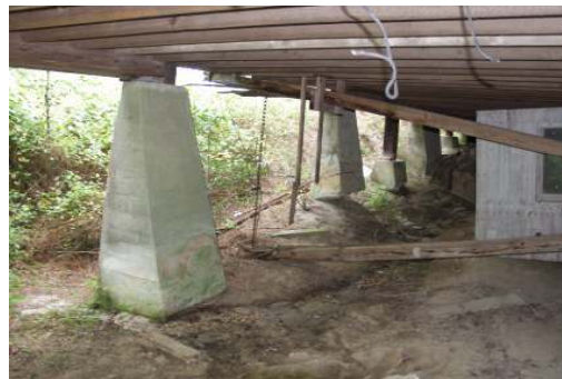
This picture shows the erosion that put the mill in danger of collapsing.
